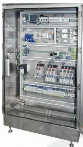
Cleverly designed electric cabinet, all cables clearly marked, reserve for future extension
